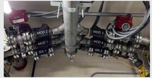
Darley's new electric valves provide enhanced efficiencies and reliability, and eliminate potential safety concerns.
