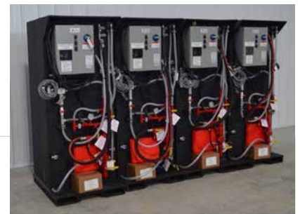
Fire protection for Mobile Housing Units.
